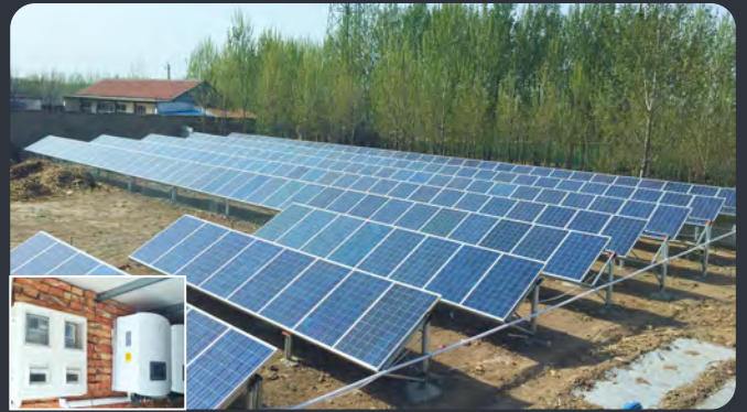
Shandong Leling poverty alleviation PV Plant | 50kW
