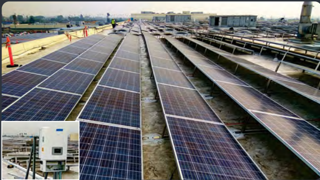
United States Postal Service (USPS) LA P&DC Facility | 12MW
