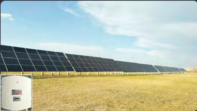
Huaneng Yimin surface mine PV plant | 20MW
