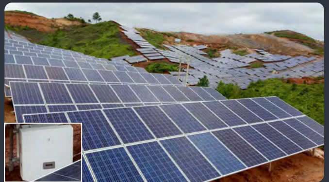
Jiangxi Ganzhou Hengjiang poverty alleviation PV Plant | 8.45MW
