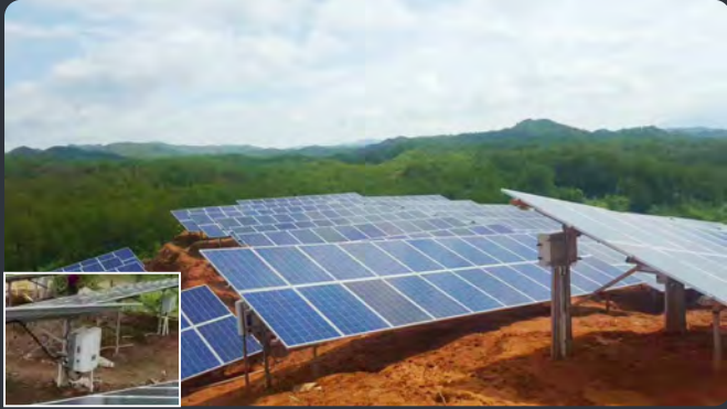
Jiangxi Shicheng poverty alleviation PV Plant | 20MW
