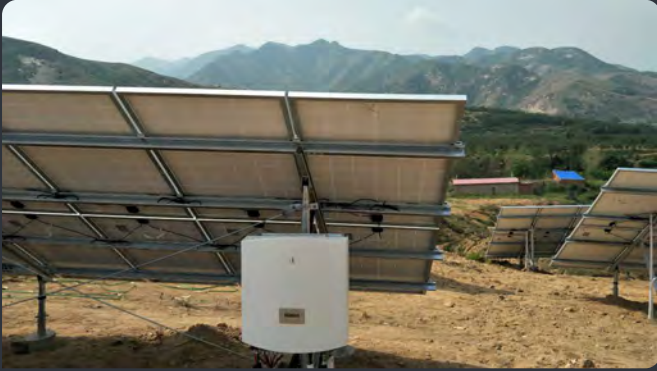
Liaoning Yingkou Jiuzhai PV plant | 20MW
