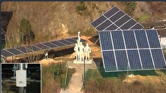
Hunan Yantouzhai Primary school | 15kW
