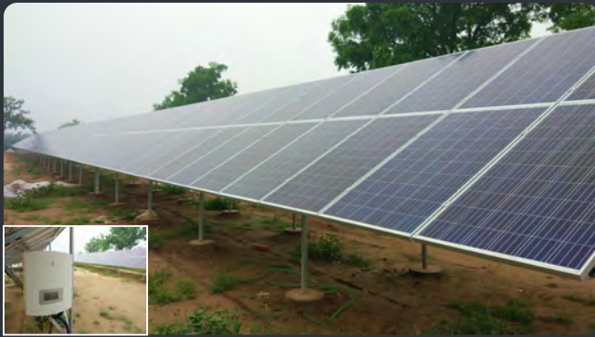
Shanxi Dazhang poverty alleviation PV Plant | 100kW
