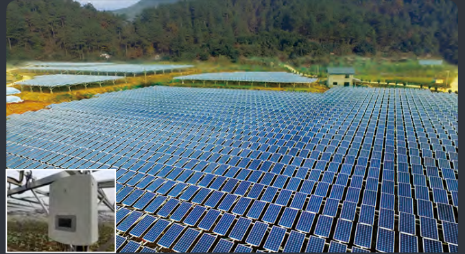
Zhejiang Dajie Agricultural-photovoltaic hybrid PV plant | 3MW
