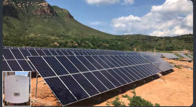
Shanxi Xiyang poverty alleviation PV Plant | 9.7MW
